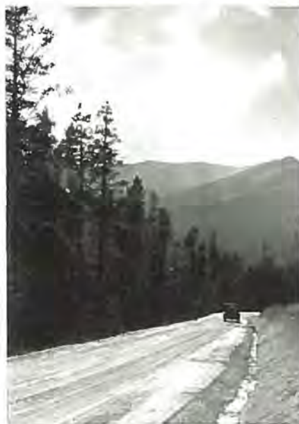
A view of the new road over Willow Creek Pass—a Federal Aid project.
