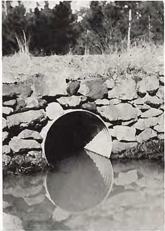
Here's an Armco Culvert placed in service in Texas in 1916. It is in excellent condition after fifteen years of service.
