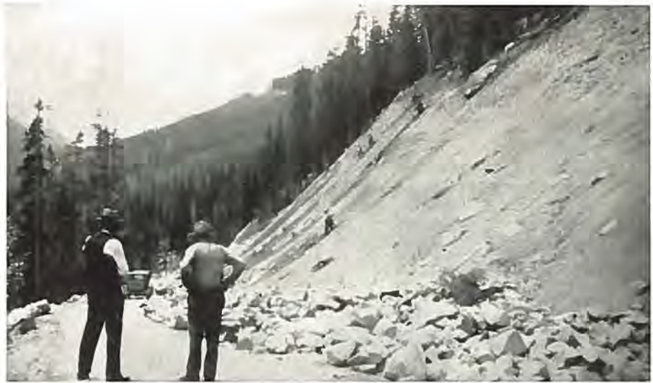
Here we have an 85-foot slope on the new Berthoud Pass highway which is nearing completion—constructed with U. S. Forest funds.
