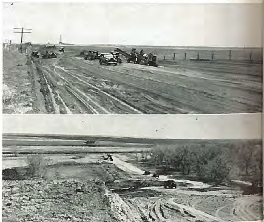
Two views showing construction operations on two sections of the Denver-Limon Federal Aid project recently opened to traffic. Photo by Roy Randall.
