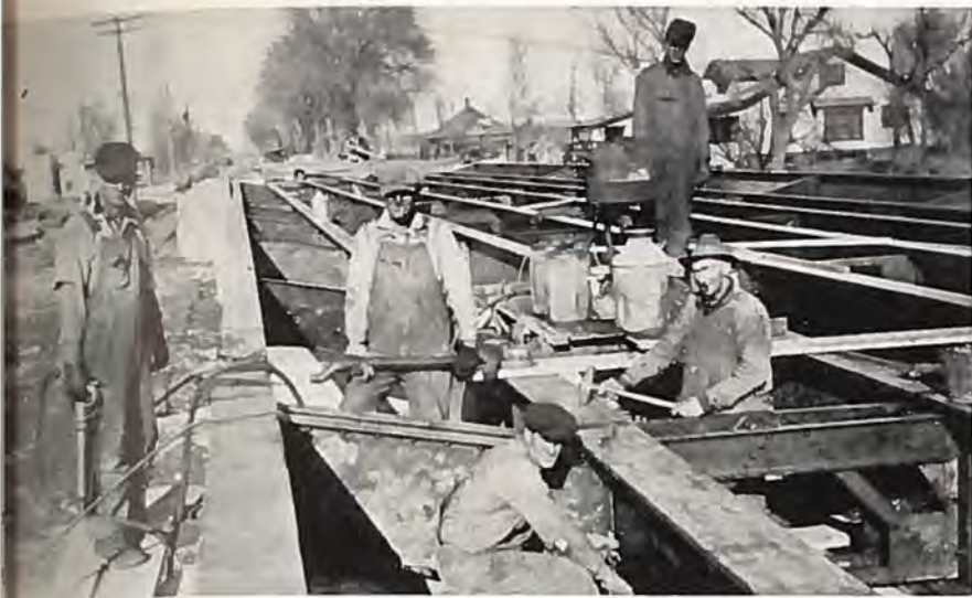
riveting 36-inch I-beams in position, making sturdy steel framework. This bridge was constructed in "dead" of winter. Photo by F. C. Dreher.
