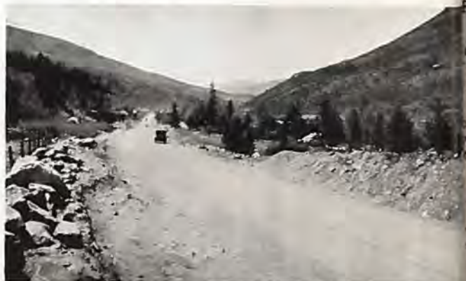
New stretch of gravel surfaced road south of Minturn recently completed with Federal Aid funds. Photo by H. L. Jenness.
