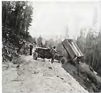
Making a fill on sidehill on the Willow Creek project, which has been converted into one of the most beautiful mountain boulevards in Colorado.
