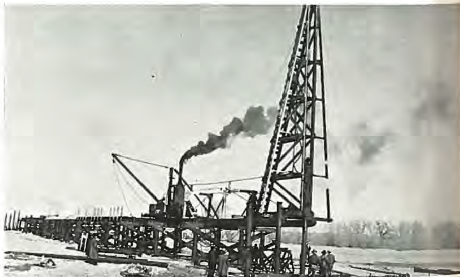
This picture shows the construction of wooden pile bridge over the Middle Bijou Creek on Denver-Limon highway. Photo by Roy Randall.
