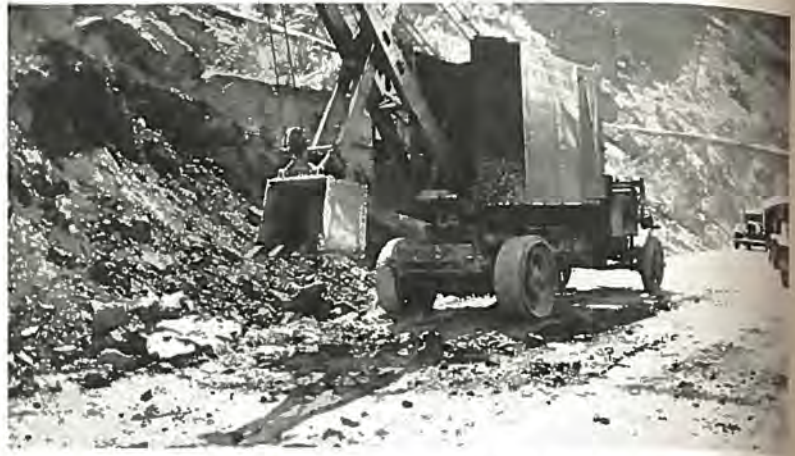
One of the State Highway Department's new Quick-Way shovels widening the road in DeBeque Canon.
