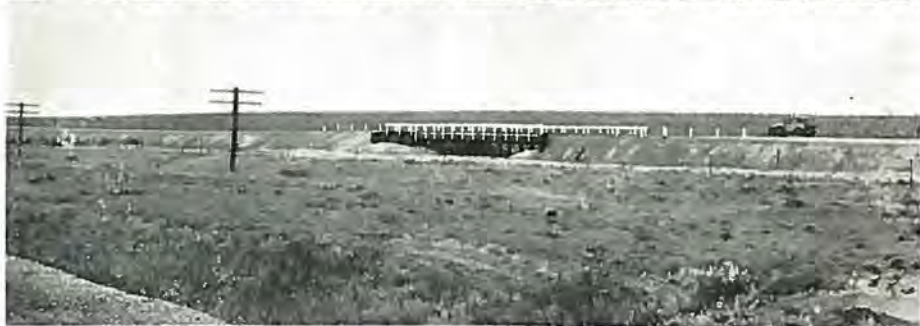
An elevating grader outfit working near Byers. One of the many wooden pile bridges constructed along the 56 miles of new roadway. Photos by Roy Randall.
