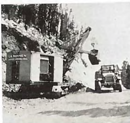
Showing a Bucyrus-Erie gas-air shovel owned by Contractor E. H. Honnen in "heavy going" on Berthoud pass, keeping a fleet of trucks busy moving excavation.
