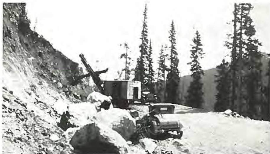
A steam shovel moving thousands of yards of dirt from the Berthoud Pass highway which is being widened and straightened by the U. S. Government.
