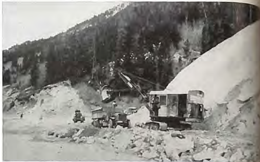
A modern shovel moving huge dirt and rock slopes from Berthoud Pass highway order to make travel over this world-famous route more easy and pleasant for the motorist. Over $500,000 is being expended by the government this summer in widening and straightening this road, which forms an important link in the Victory highway.
