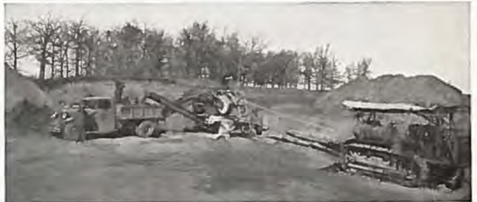
This shows the complete hookup of Fred Hillquist's No. 22 Pioneer Plant with power unit. Delivery conveyor is loading truck.
