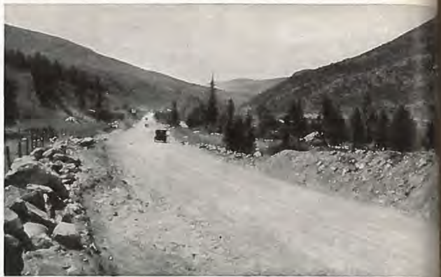
An example of gravel surfaced highway constructed near Avon in Eagle County, struced under Federal Aid specifications. Photo by H. L. Jenness.
