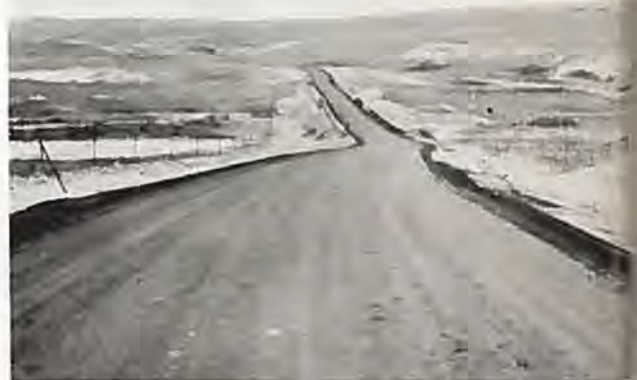
Showing a stretch of oil processed highway northwest of Fort Collins near Virginia Dale.
