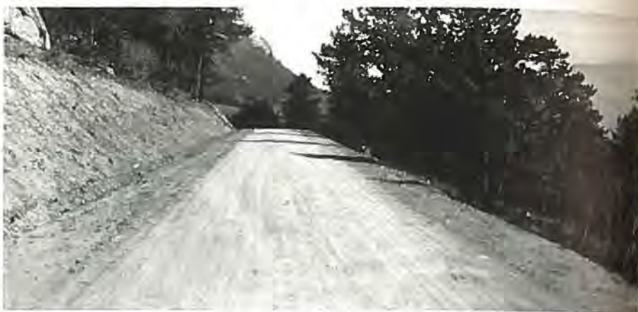
Showing a section of the new road being constructed by the Forest Service over Willow Creek Pass, leading into the North Park country from the Colorado River, near Granby.
