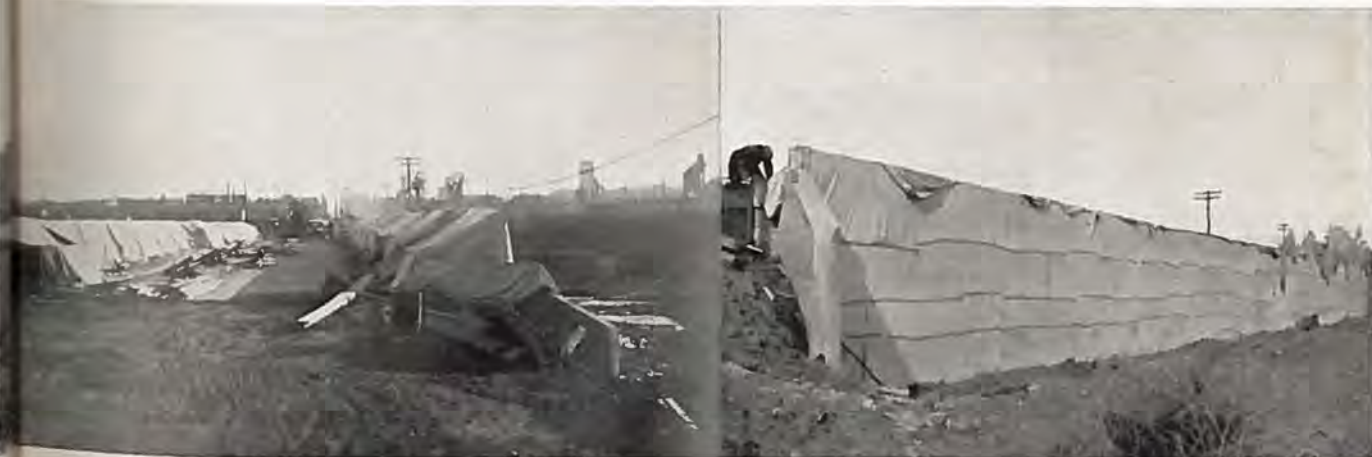
Two pictures showing method employed to prevent freezing of concrete. (Left) Hand rail protection against freezing. (Right) Bridge enclosed with canvas against freezing. Photos by F. C. Dreher.
