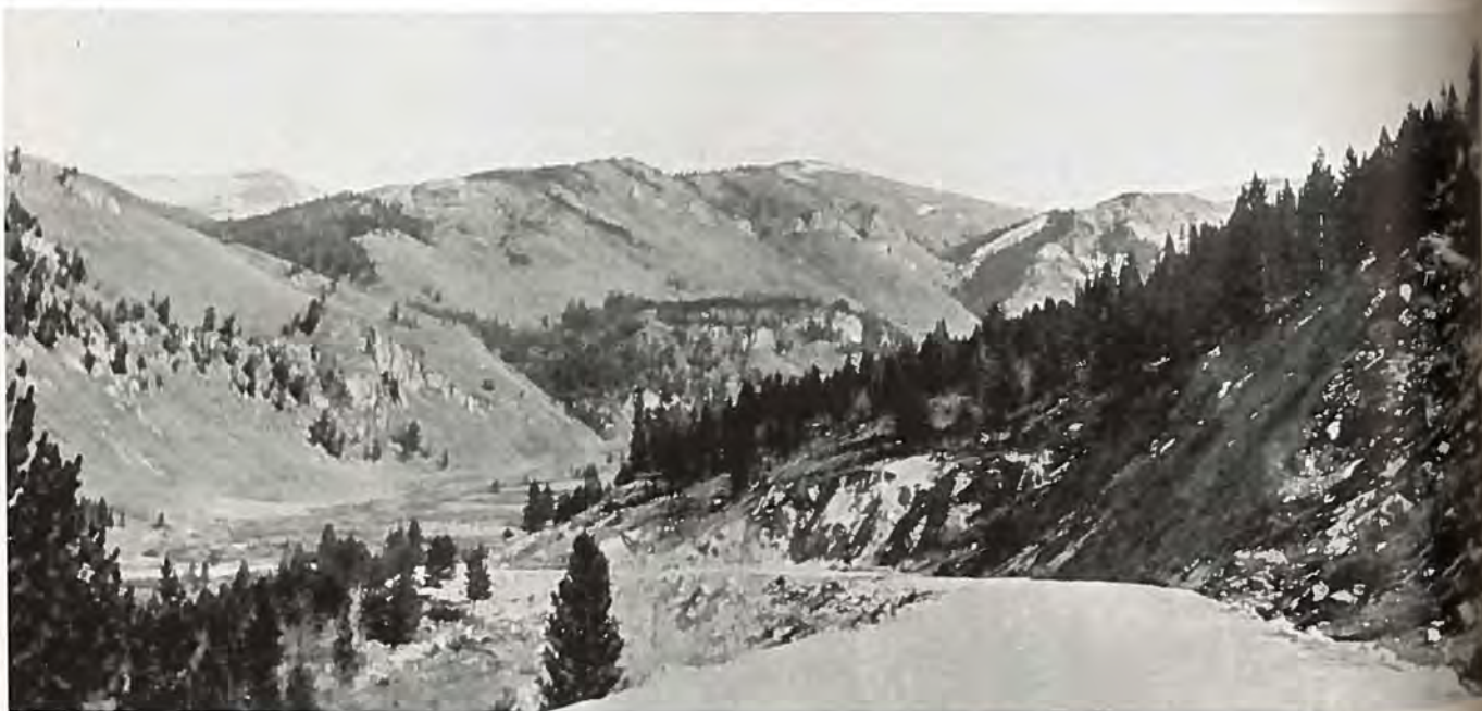
Finished road after application of crushed rock surfacing, where several sharp curves and steep grades on old road were eliminated.
