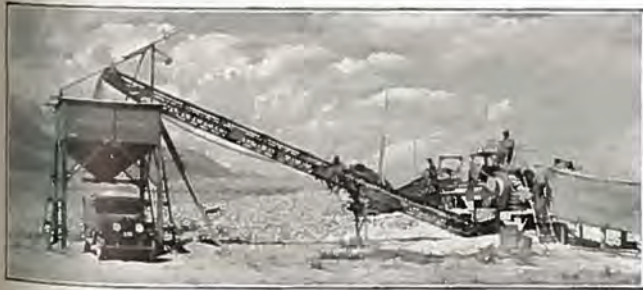
No. 12B Pioneer Screening, Crushing and Loading Plant owned by Threet Bros., Lovell, Wyoming, operating in Teton mountains in Wyoming and producing large daily capacities
